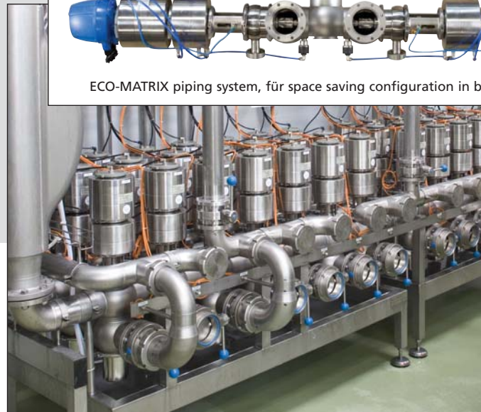
Valve matrix with VARIVENT® mixproof valves in a dairy plant
