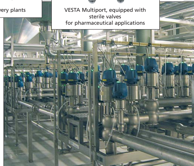
Valve matrix with VARIVENT® mixproof valves and T.VIS® control modules installed in a brewery
