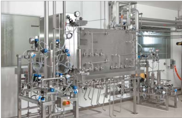
The media panel forms the central interface between all pipes in the formulation area and the pipes to the product tanks, it also accommodates all CIP and SIP connections.
